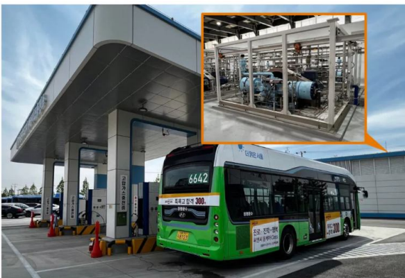
PDC Diaphragm compressors (Seoul Bus Terminal)
