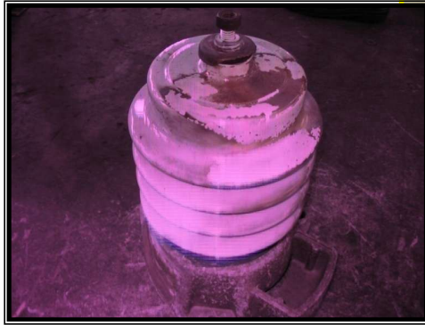
避雷器故障損毀
