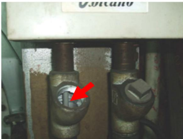
電管密封配件內部未填塞防爆泥
